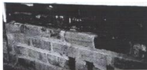
Fig. 28 Base of the dining room wall, La Trobe's Cottage, showing the wall plate and the bases of the studs, photograph, Miles Lewis.
