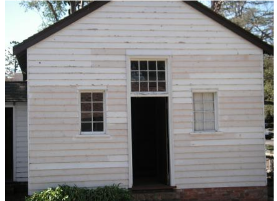
New timbers installed at the Servants' Quarters. Hailstorm damage is evident on old timbers
